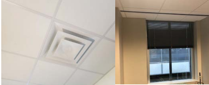
Picture 2: Alnor Balometer Set-up and Measurement Using 2x2 Capture Hood (Left) and Slot Capture Hood (Right)
